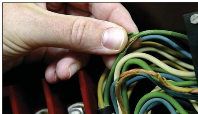
Aging and ionizing radiation degrades the insulation on the PS dipoles' pole-face winding. This is one reason for the renovation.
