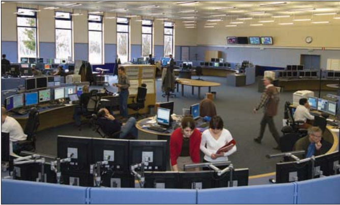
The new CERN Control Centre unites all the control rooms.
